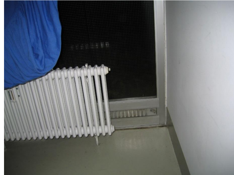
Paint in the laundry-room of an apartment building: Paint on screed (floor) and plaster (wall)
