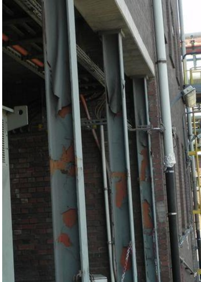
Flaking anti-corrosion paint
