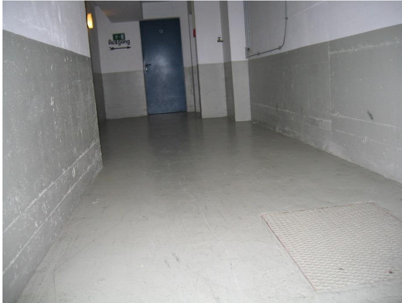
Paint in the basement of an apartment building Paint on concrete (floor, walls), paint on fire protection door
