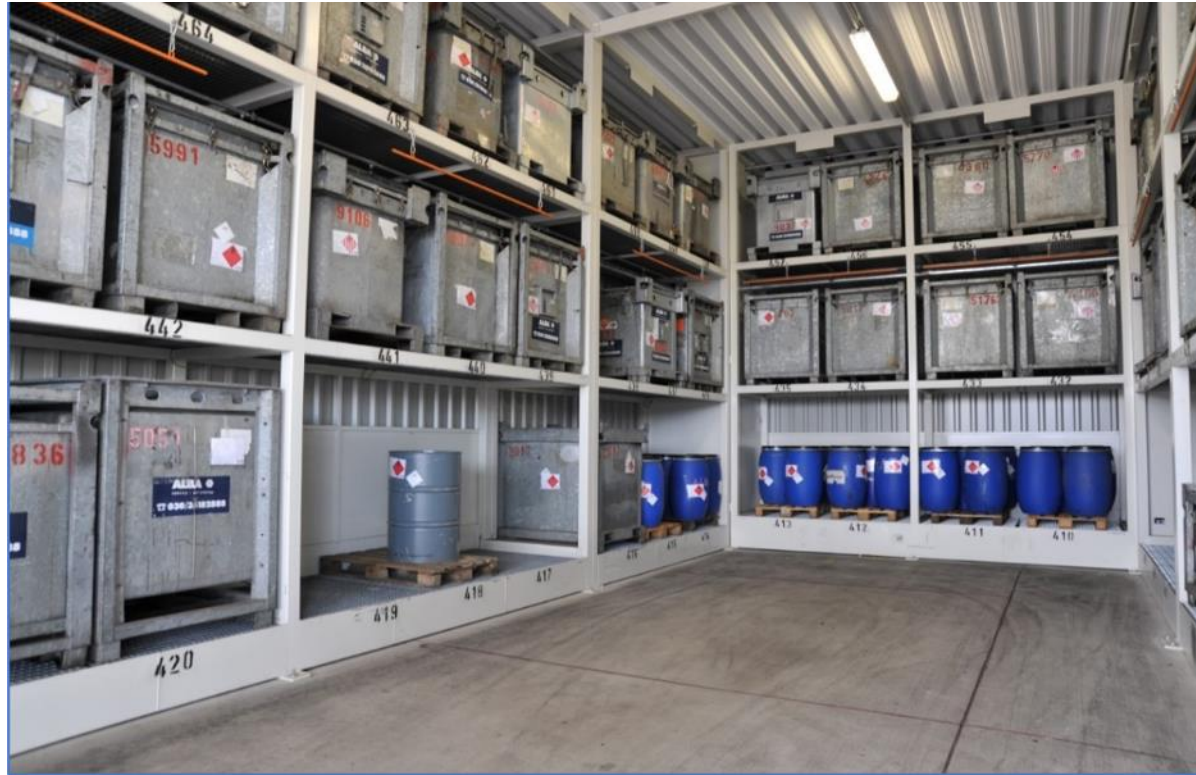
Centralised Hazardous Waste Storage Facility in Germany, e-g- TRGS 510
