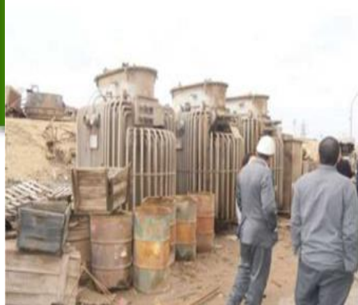
Picture 7: Transformer No 1
